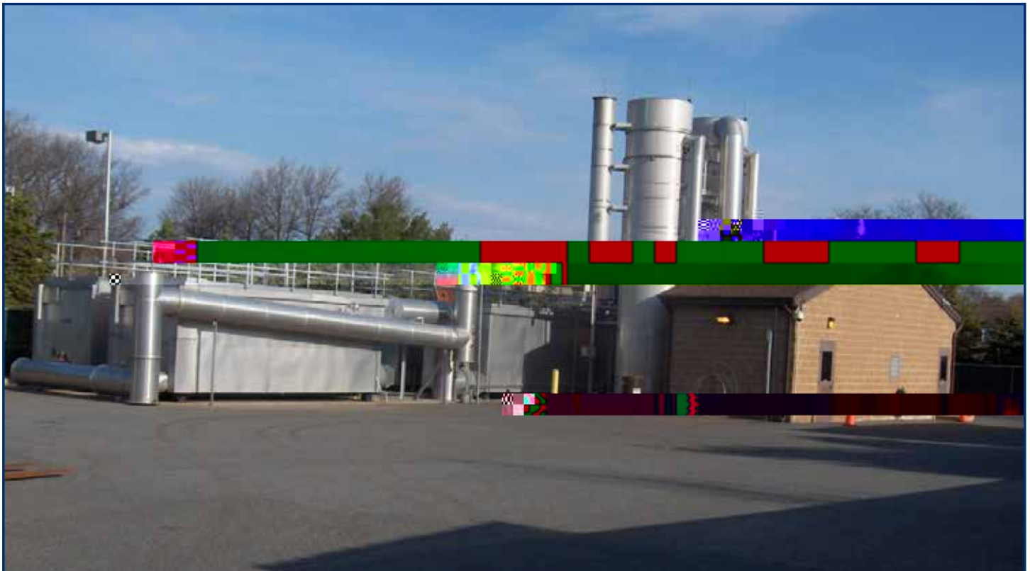
On-Site (OU1) Groundwater Treatment System
